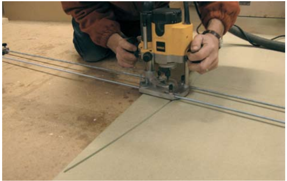
2 Working on the floor to cut the leg template using router and trammel
