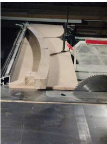
4 The end of the back legs are trimmed at the correct angle using a jig on the tablesaw
