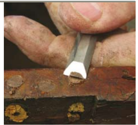
2 Trimming off the dowels inserted to strengthen repair to left of flap
